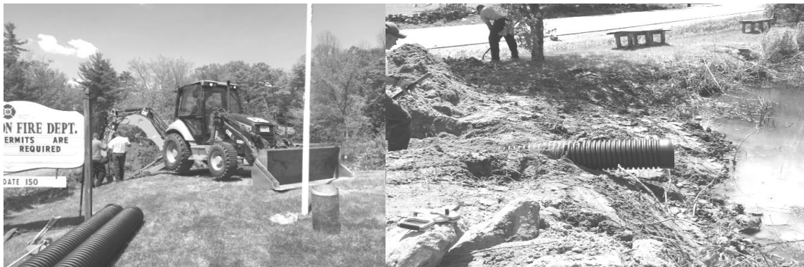
- The Highway Crew assisting with repairing the Fire Pond in the Square -
