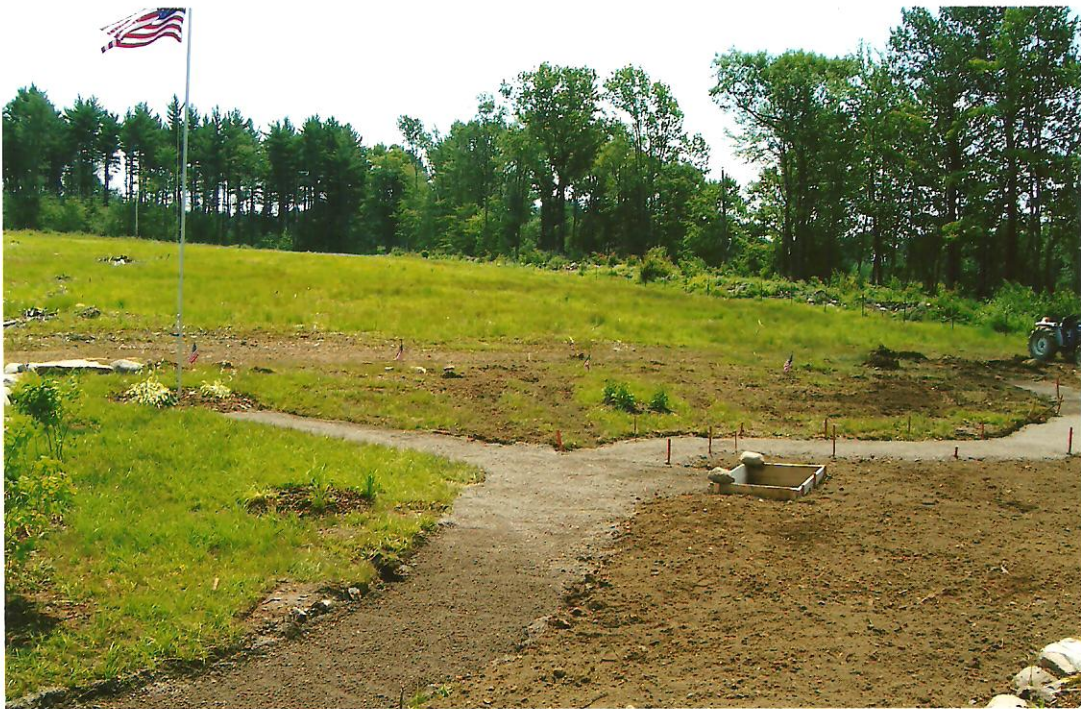
Stone-Dust Laid On Pathway & Ready To Concrete The Bench Base. The Latham's Donated A Compactor For The Pathway
